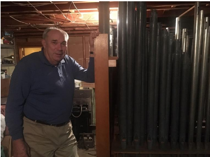
Bill Johnson next to the pipes for the Estey organ installed in his basement.
